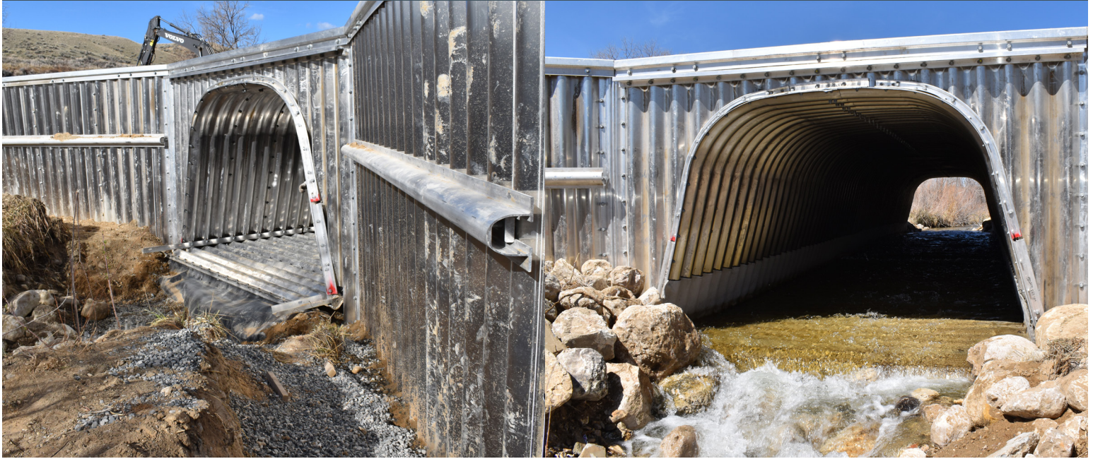
Cody, WY culvert before RCR® remediation
